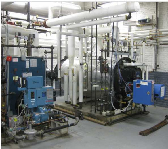
AEA Heating and Cooling Laboratory Featuring fully functional Multifamily boiler systems
